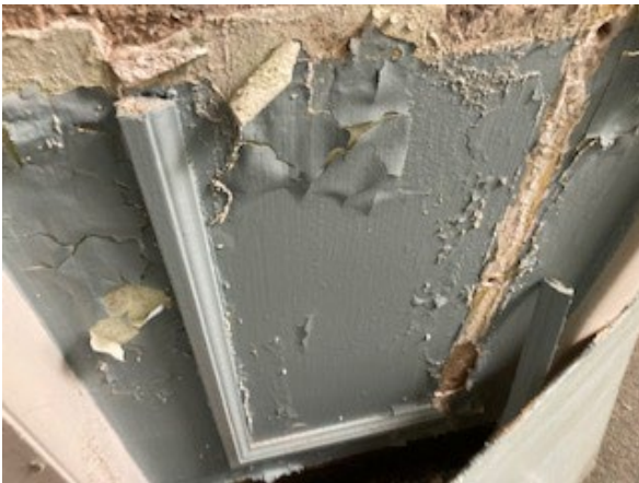
Evidence of prior bathroom leak.
