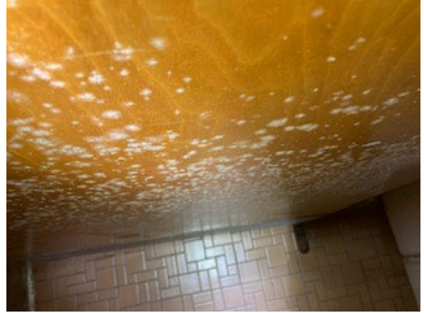
Probable mold on door.
