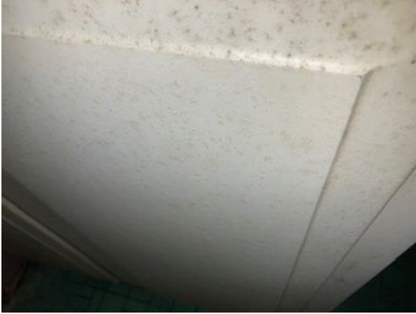
Probable mold on cabinet.
