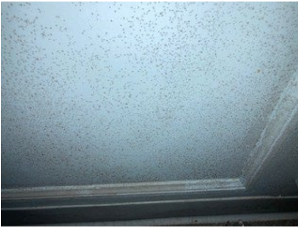
Probable mold on wall.
