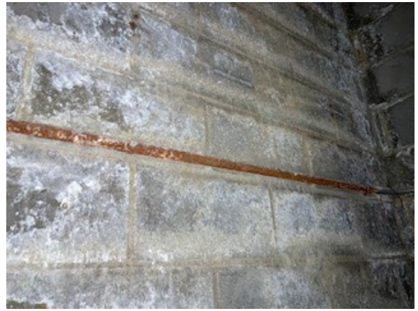
Efflorescence on furnace room wall.
